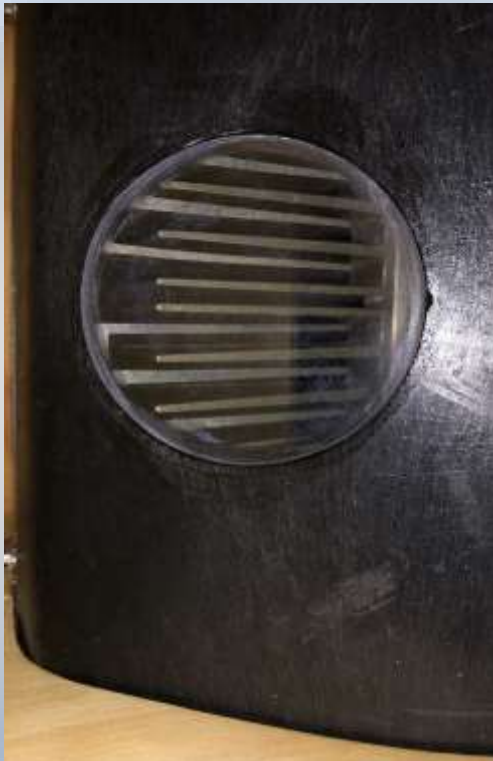
Looking into left window with capacitor fins fully meshed.
